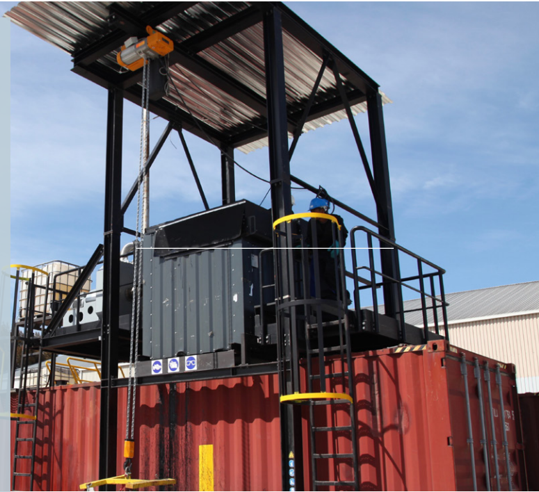
High-Performance Melter - Melting Site / South Africa
