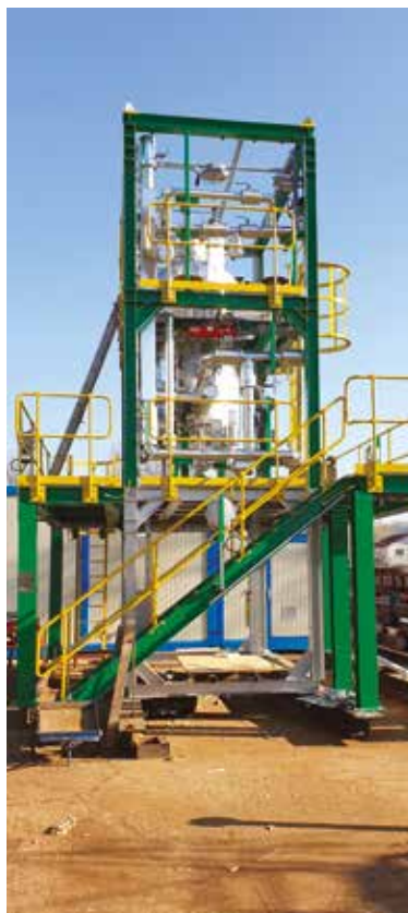
The skid-mounted Bolashak Onshore Processing Facility (OPF) is located near Atyrau, where oil and gas from the offshore Kashagan field is processed.
